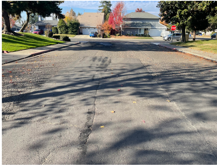
Photo 4: Andre Lane Patches (Patches and Failed Pavement)
