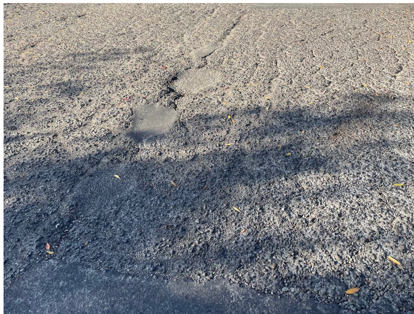
Photo 3: Regis Street (High Severity Alligator Cracks, Potholes, and Raveling)
