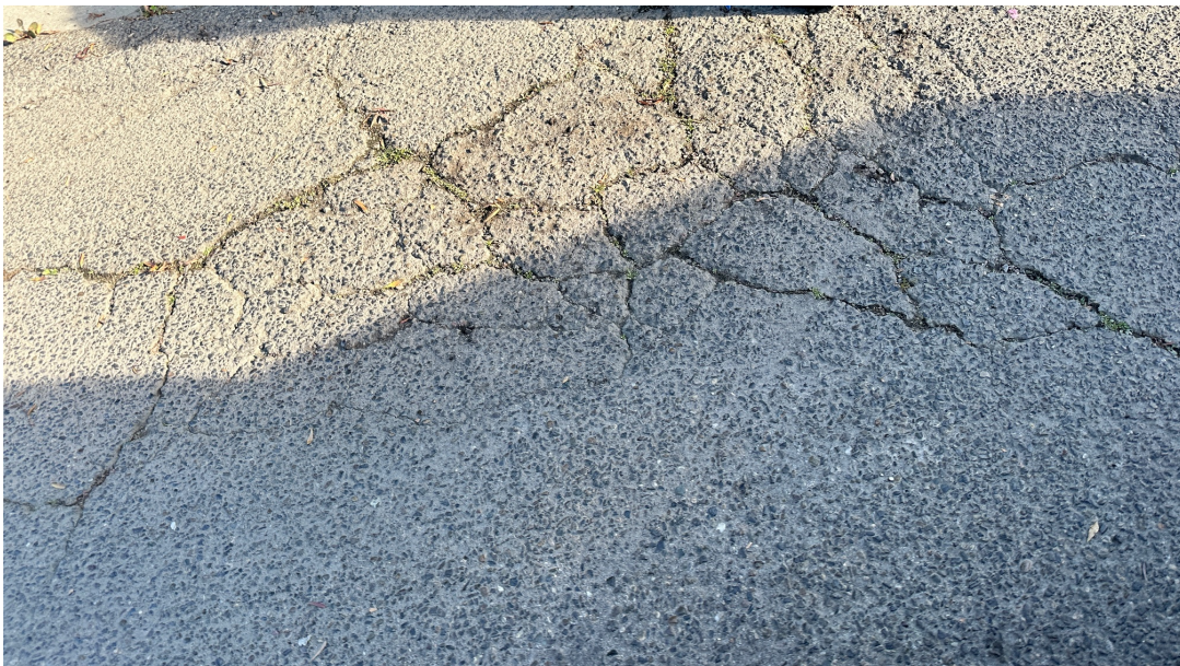
Photo 1: Curt Court (Alligator Cracks)
